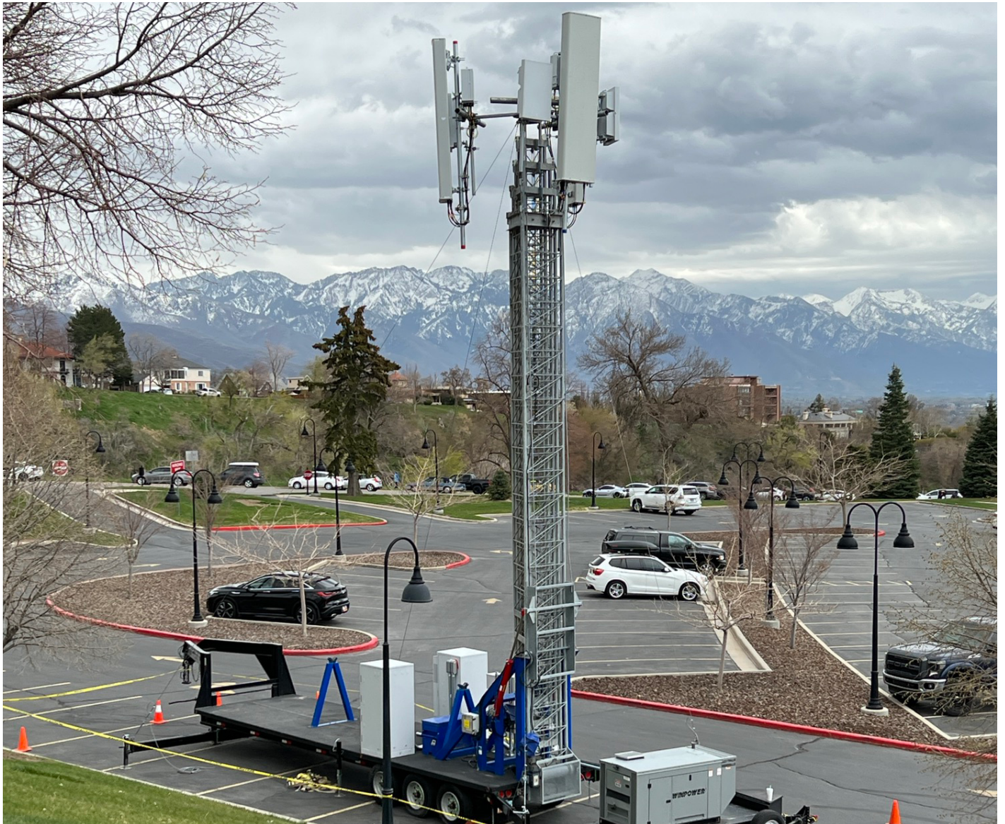
Mobile Cellular Tower in Salt Lake City, courtesy of Imgur
